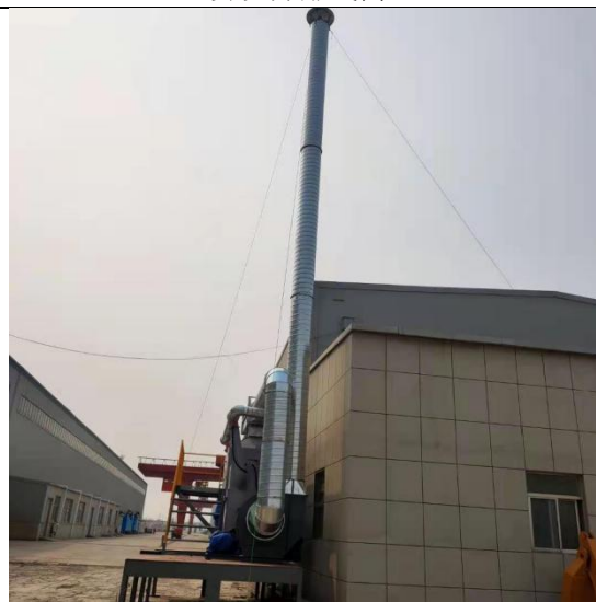
喷漆房排气筒
